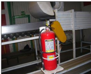
Photo of fire safety equipment Fire extinguisher.JPG
