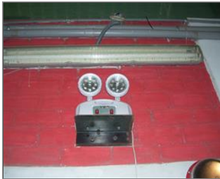
Photo of fire safety equipment Emergency light.JPG
