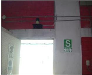
Photo of fire safety equipment Emergency exit door.JPG
