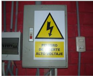
Photo of the inside of the main production hall Warning signs on electrical panel.JPG
