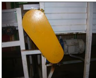
Photo of the personal protection equipments (if applicable) Safety guard for machinery.JPG
